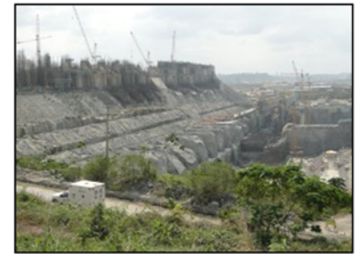
The Belo Monte hydropower complex. Photo credit: Dr. Kirk Winemiller, Texas A&M University
